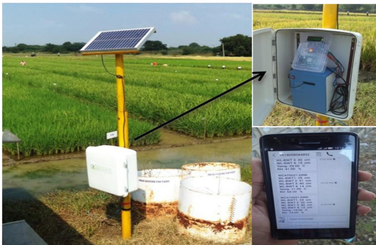
Figure 3 A smart irrigation device installed in the field (Adopted from Mallareddy et al., 2023)
